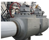
Double Block & Bleed VV
